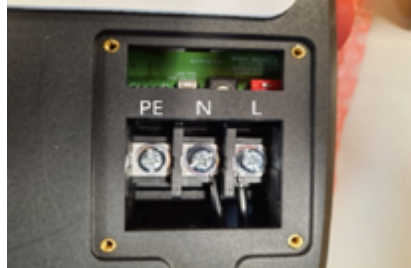
Terminals inside the charger (on the back of the charger)
