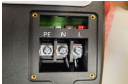
Terminals inside the charger (on the back of the charger)
